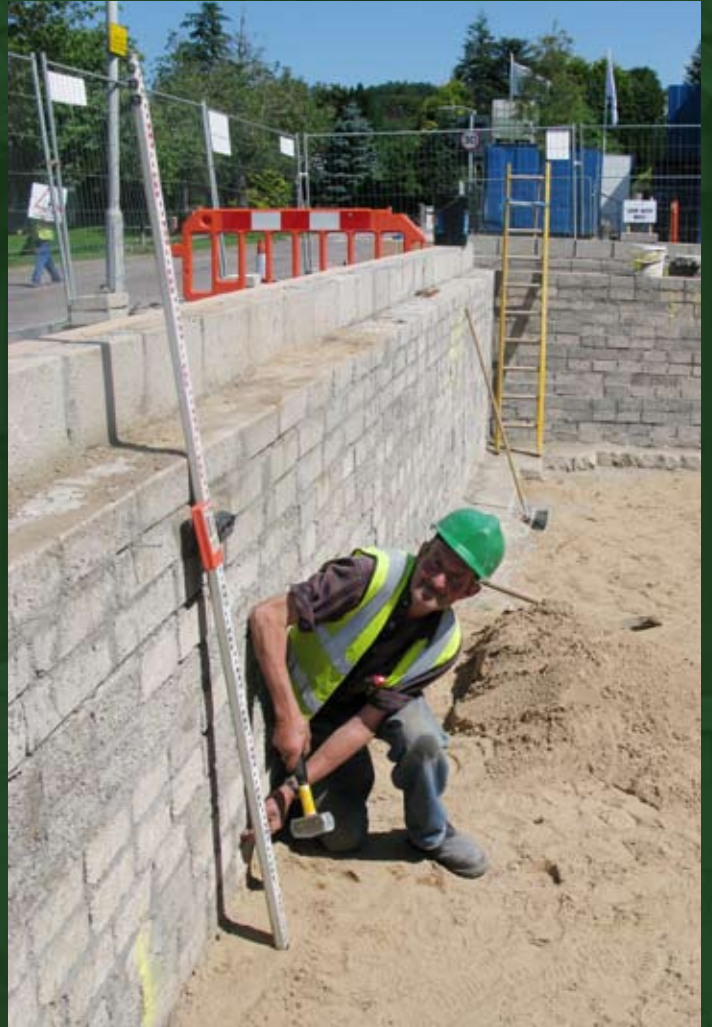
Springfield labourer Norman McLeod busy in the pool pit as the Moray Hydrotherapy Pool takes shape alongside Forres Swimming Pool.
