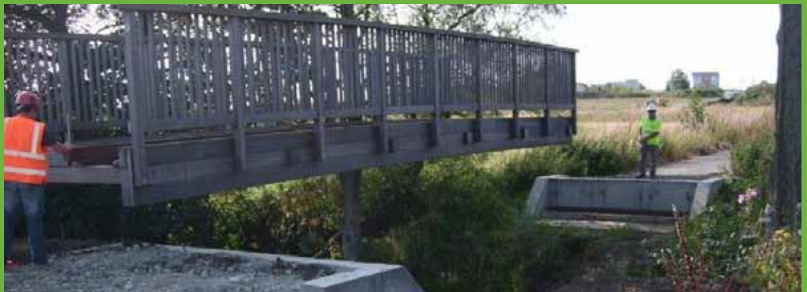
Gently does it! This timber bridge being lowered into position at our Middlebank Rise development at Dunfermline was a planning consent requirement. It links into all of the new paths which form the walkways, cycleways and safe routes to school and other facilities and run through the extensive Dulloch area. The 12 metre long wooden bridge was made in Holland and weighs six tonnes and needed a 240-tonne crane to lift it into position and carefully locate it on its base.
